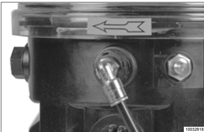
Fig. 15- Return line connection
